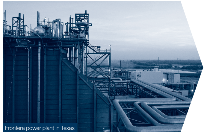
Frontera power plant in Texas
