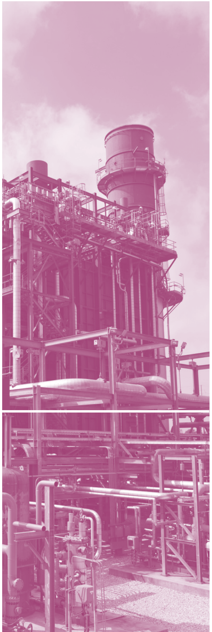
Bastrop Energy Center, Texas, United States of America
