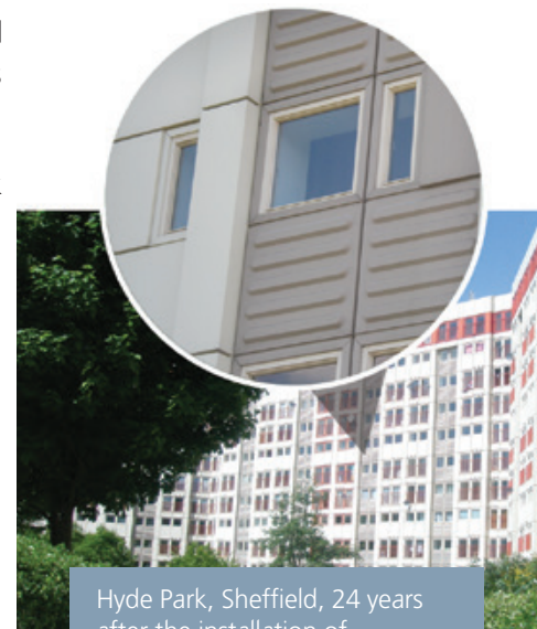
Getting it wrong – 6 years after the installation of a board system
